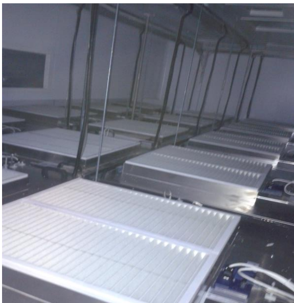
Picture showing a recently installed Fan Filter Unit project walk on ceiling (Plenum side view)
